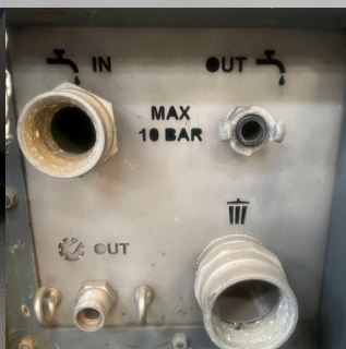
Water inlet and outlet
